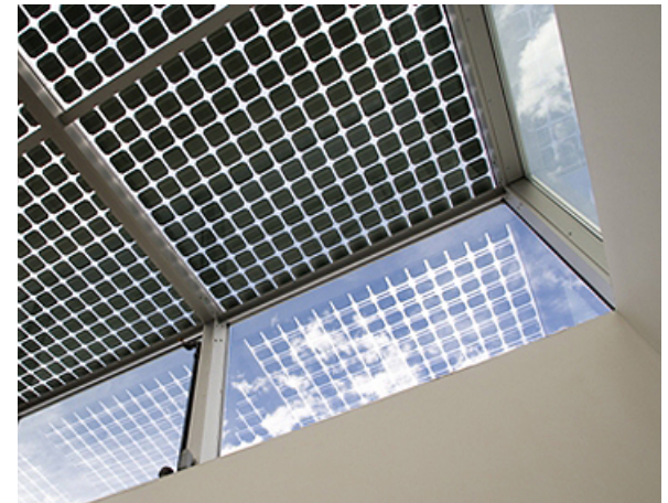
Building Integrated PV
